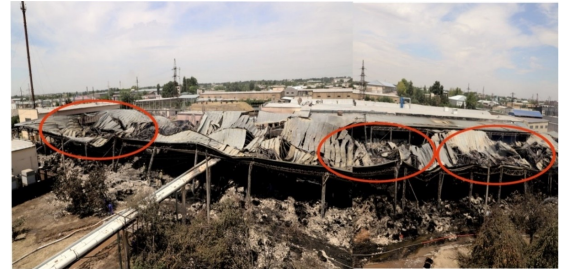
Fig. 1. As a result of the emergency situation, the structure of the building changed its shape and the most damaged areas
